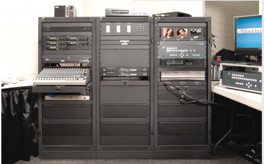
The equipment rack plus a switcher Novatoo added for the annual meeting.
